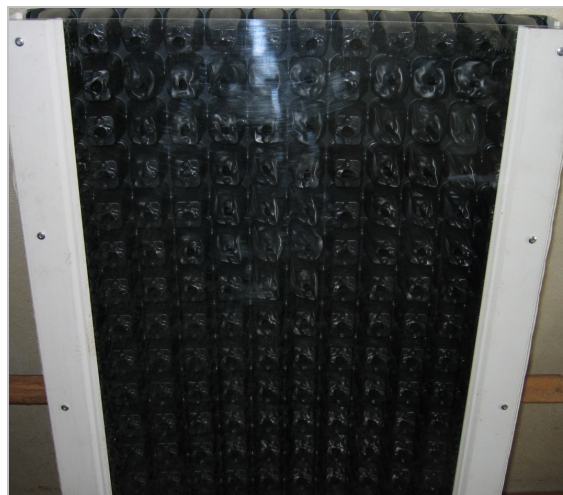
Fig. 7 Absorber defect in air heating sun collector in very good weather conditions
