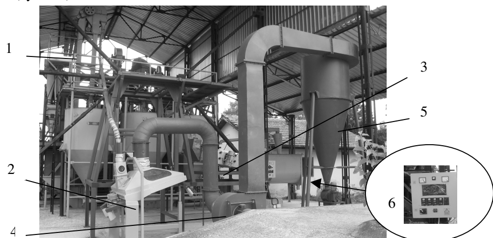
Fig. 3. General view of the installation used in experimental research: 1 – elevator; 2 – gravity separator; 3 – intensive vacuum separator; 4 – fan, 5 – dedusting cyclone; 6 – control and signaling panel
