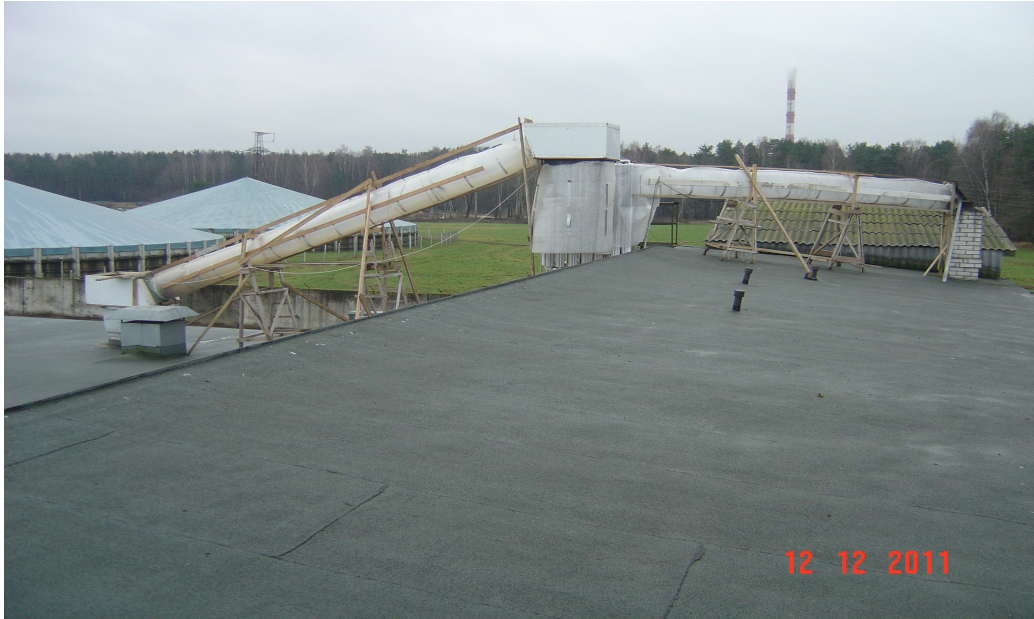
Fig.1. Heat pump evaporators covered by special screens (in the centre), warm air fanned tube from the piglets room (on the left) and flue gas fanned tube from the chimney of the farm boiler house (on the right)
