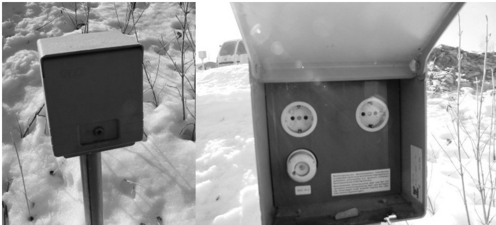
Fig. 5. Sockets for engine heating in town Nokia, Finland
