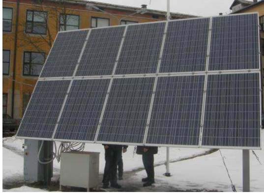
Fig. 2. Two kilowatts PV array of 10 Kyoto KPV 195 PE modules
